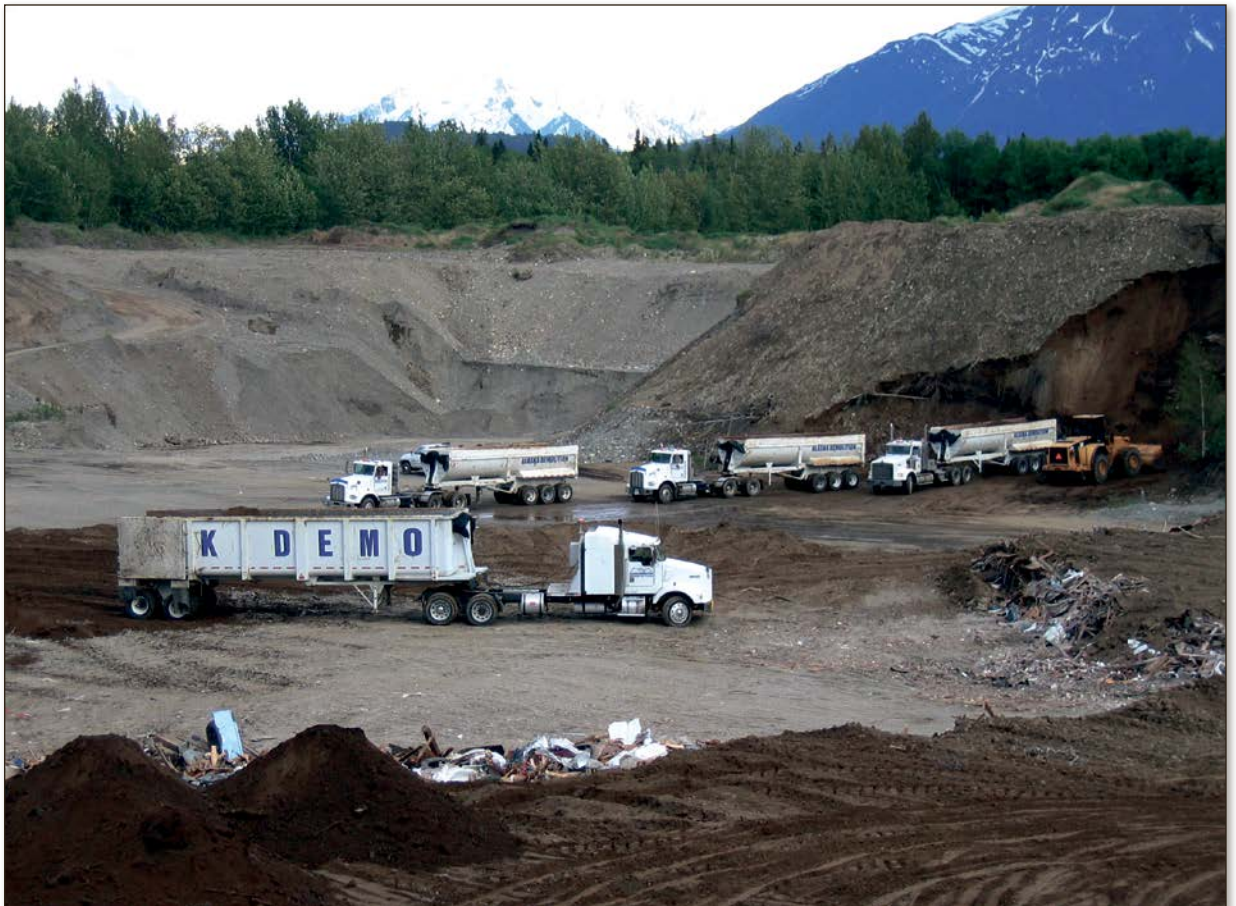
Disposal transport tractor-trailers line up at Alaska Demolition's 38-acre reclamation site in Palmer.
